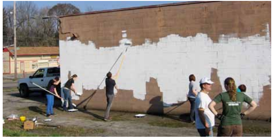
Assisting in the preparation of a wall for a new artistic mural in Youngstown's Idora neighborhood. Photo Credit: Marianne Eppig
